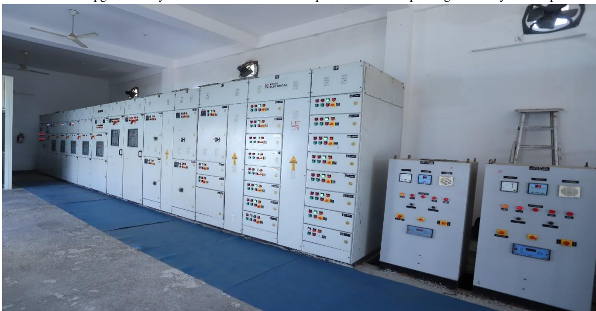
IPS Control Panels, Ghaziabad
